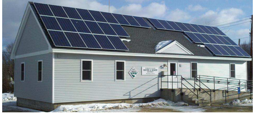
Office building retrofitted as a net-zero energy building. Project added 4" of insulation for energy reduction plus 9 KW of solar photo-voltaic panels for electric generation (PV installation by Revision Energy of Liberty, Maine).
